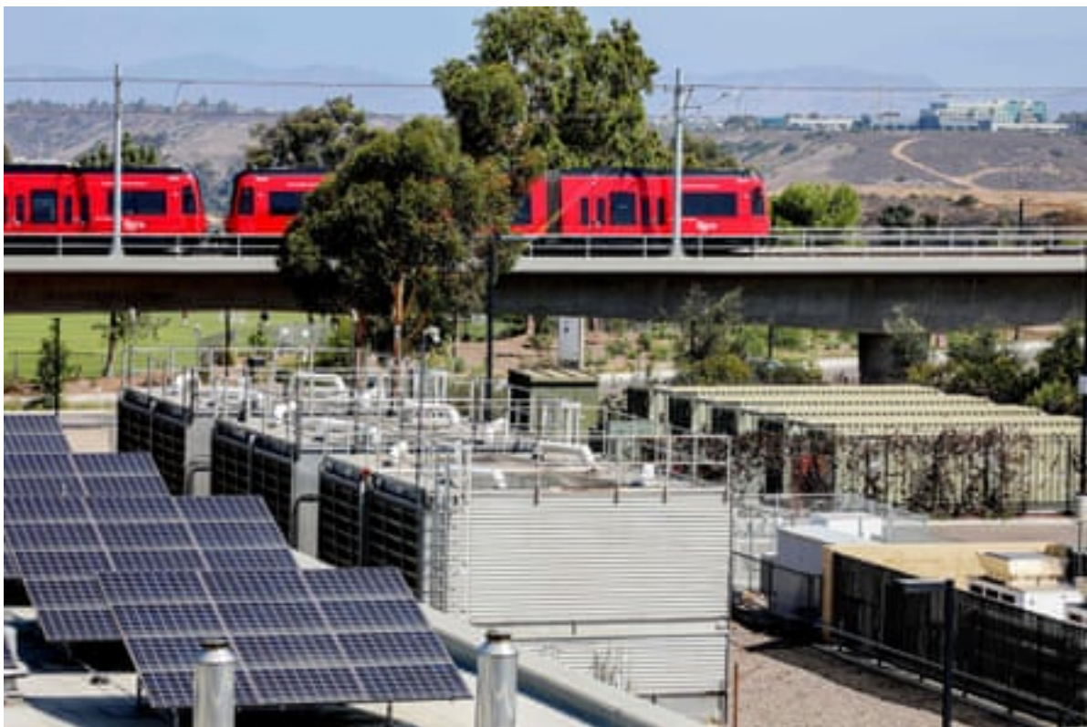
Energy storage containers with lithium ion batteries (right) at the University of California San Diego. Photograph: Sandy Huffaker/AFP/Getty Images
