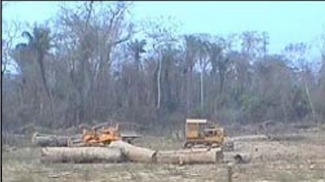
Bulldozers are used both to drag logs and to forcibly clear areas of vegetation. These were being used to do both.
