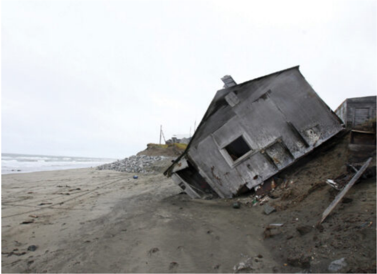
Beach erosion destroyed this home in Shishmaref, Alaska, shown in 2006; now the whole village must move because of sea level rise.
