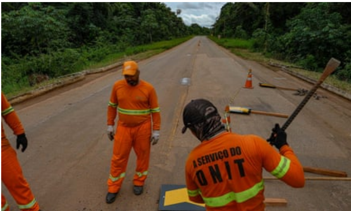
Workers carry out maintenance on a paved stretch of the BR-319. Photograph: Alberto Cesar Araujo/Amazônia Real
